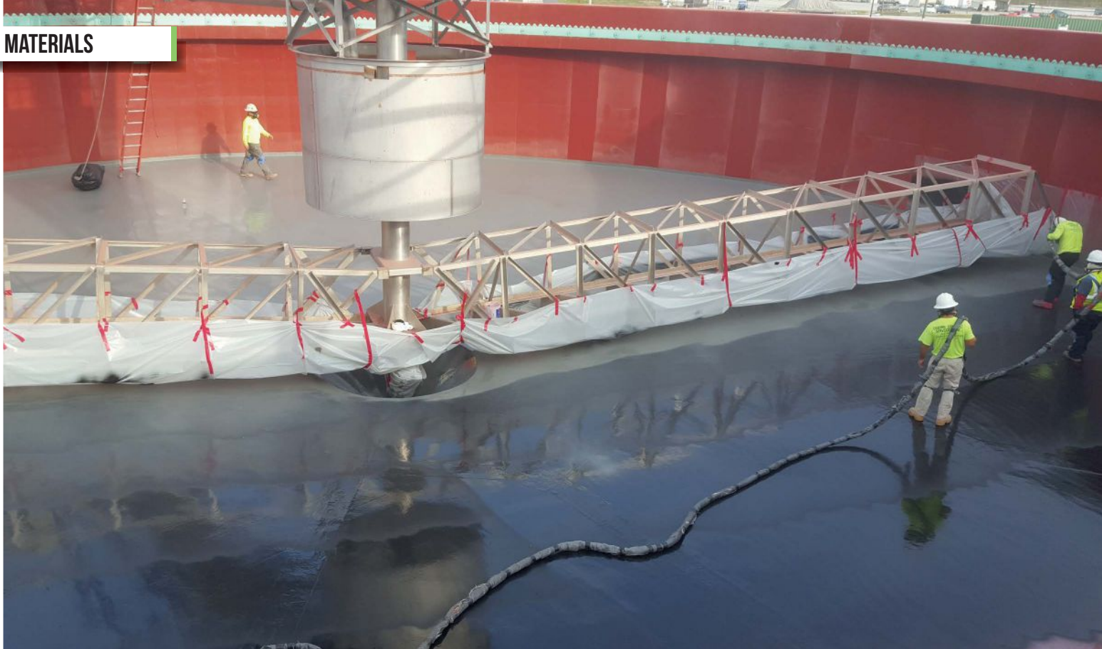
Spray-applied polyurea coatings create a seamless, waterproof, durable protective liner that stops leaks and strengthens the integrity of the entire structure.
