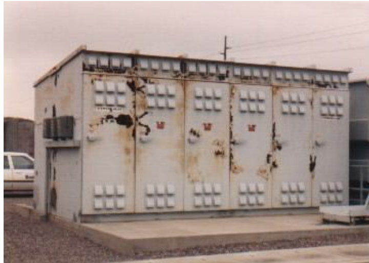
Typical Chloride Induced Coating Failure
