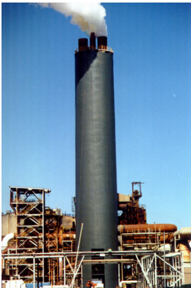
Below: Finished installation of FSS 45DC
