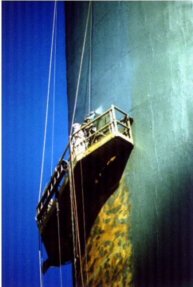
Above: Workers brave 40mph winds while hanging hundreds of feet above the ground.
