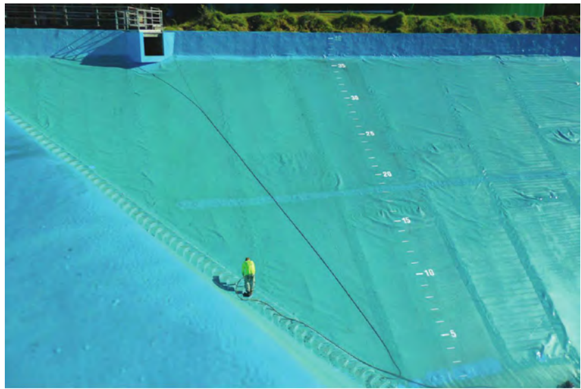
To provide cost-effective, decades-long waterproofing restoration the restoration contractor used pre-sprayed composite panel system combining geotextile and a pure polyurea membrane from VersaFlex.
